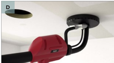
Sand joints: Sand the filled joints with your preferred tool to level the panel surface.
