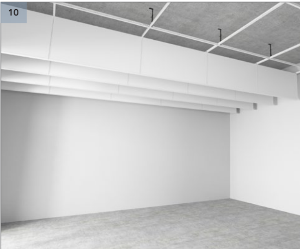
Fix all the remaining Rockfon Humitec Baffles to the T24 ECR grid and align.
