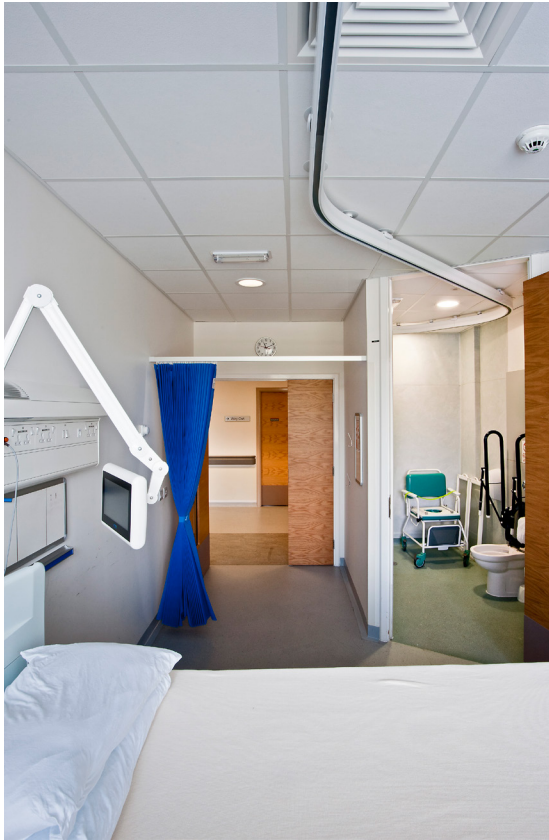
Installer Linear Projects Ltd Products Rockfon® MediCare® Standard, Rockfon® MediCare® Plus, Chicago Metallic™ T24 Click D2890 ECR Class D
