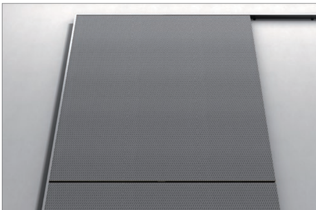
3.5 Install any intermediate panels, working from the uppermost to lowermost side of the panel. They should sit securely in place via supporting bracket(s) and the J-channel – see diagram on page 6.
